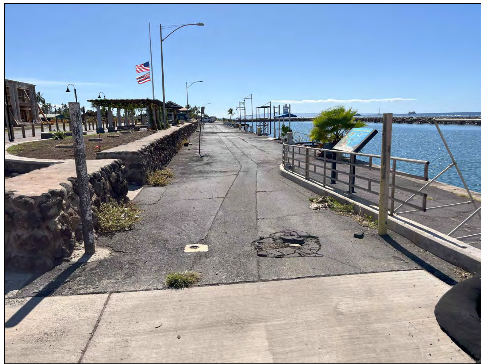
2 EXIST. RAMP (NORTHERN END OF LAHAINA SBH) TAKEN 01/21/2025
