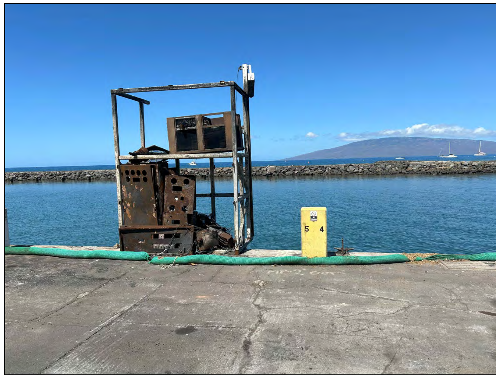
2 EXIST. METAL STRUCTURE & DEBRIS TO BE REMOVED TAKEN 06/25/2024
