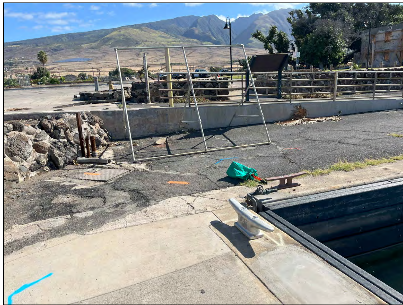
1 EXIST. CONCRETE WALL AND HANDRAIL TO REMAIN ON NORTHERN SIDE OF LAHAINA SBH, FRONT ROW TAKEN 01/21/2025
